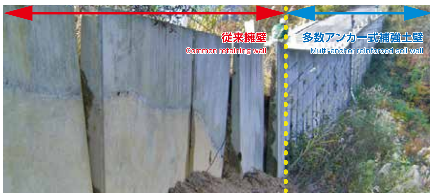
被害が発生した従来擁壁(左手前)と、持ちこたえた多数アンカー式補強土壁(右奥)。Common retaining wall that suffered damage (left side, toward the front), and a multi-anchor reinforced soil wall that held up (right side, toward the rear).
